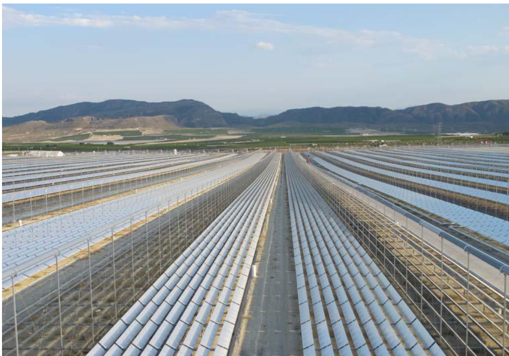
30 MWe Puerto Errado-2 (Murcia), by Novatec
